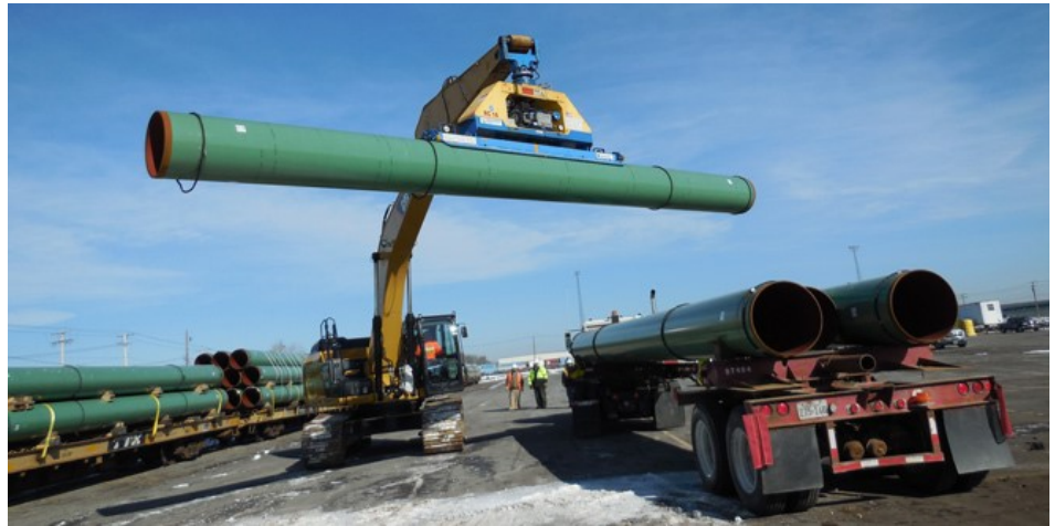
The first sections of the Constitution Pipeline arrive in New York. Source: Constitution Pipeline
